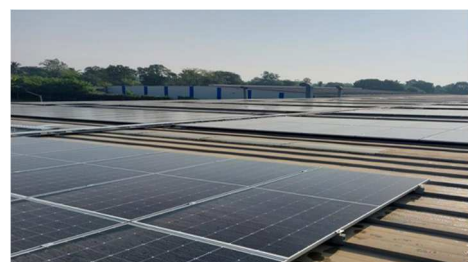
Solar panels to improve energy efficiency in plant
